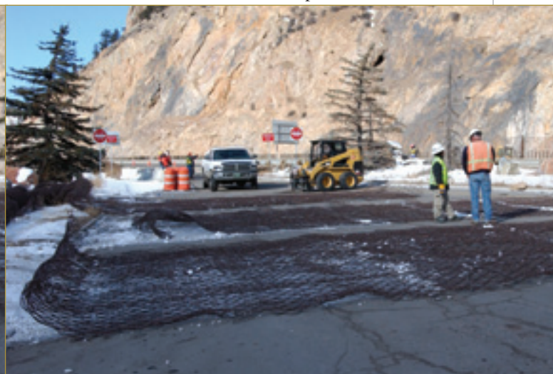
A worker reaches for the spreader beam that will be used to hoist the mesh section. Keeping the mesh spread out as it's picked up by helicopter is tricky.
