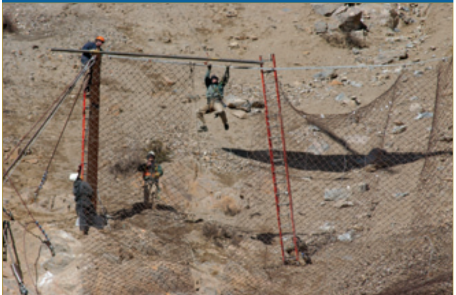
Above: From their precarious perch on the mountainside, ground crew members dangle as they secure the mesh.
