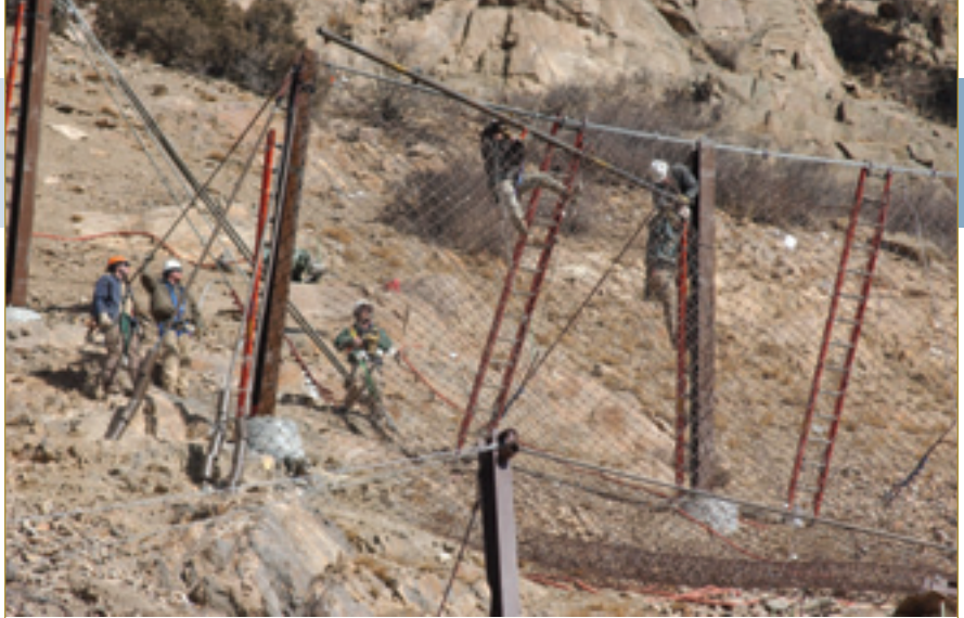
Above: Crews secure the 1,200-pound piece of mesh into a huge chain link fence. This extra-strong mesh is similar to chain link mesh used underwater by the military to seize submarines.
