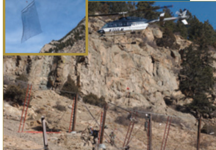
At the installation site, the crews on the ground grabbed a tagline to maneuver the mesh into place and attach it to the
